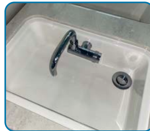
Galley - Freshwater Sink with Pullout Shower
